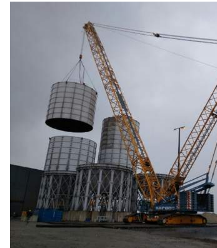
SILO CAPACITY: 5.000 ton DIAMETER: 14,6 m HEIGHT: 43,8 m
